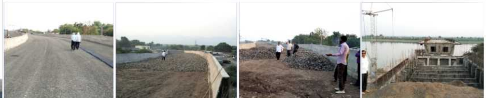
Tapi river Major Bridge, approach road, under pass, protection wall At Hatoda Village, Maharashtra- Gujrat State Border
